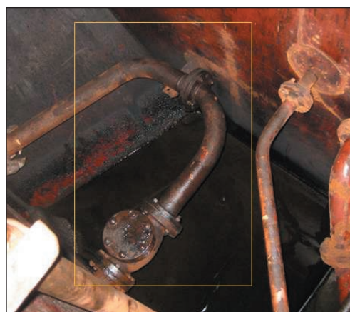
The hose used to bypass pollution prevention systems was connected here after this section of piping was removed. USCG photo.
