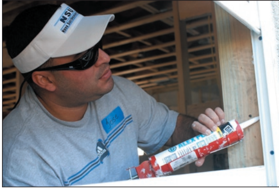
Petty Officer 2 nd Class Jose Urbina of the Naval Engineering Support Unit at Sector Miami caulks a window at a Habitat for Humanity home being built in the Scott-Carver neighborhood of Miami. Coast Guard volunteers devoted 10 days of their time and energy helping to finish up the final 10 of 52 homes built in the Scott-Carver neighborhood.
